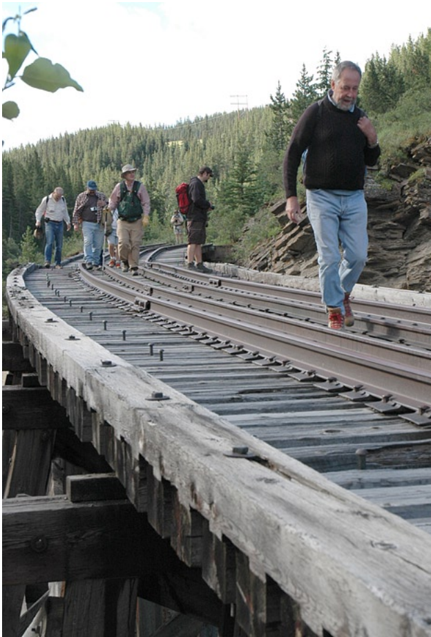
Field trippers negotiate one of the wooden trestles on the abandoned Cadomin-Mountain Park line.
