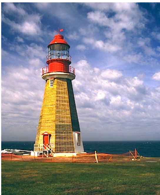
Figure 18. Point Riche Lighthouse is an active “pepper-pot” (salt and pepper shaker shaped) structure standing tall at 19 metres (62 feet) since it was first built in 1892. This rare shot of it was taken while its exterior was under renovation.
